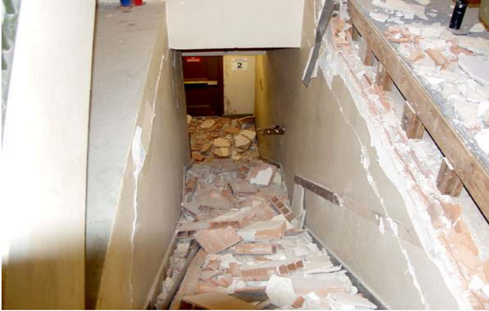
Damaged courthouse stairwell, King County, Washington Nisqually earthquake, February 28, 2001. (Photo courtesy King County, Washington State.)
