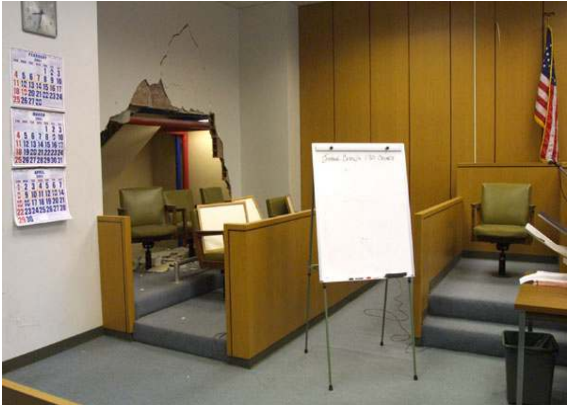
Damaged courtroom, King County, Washington Nisqually earthquake, February 28, 2001. (Photo courtesy King County, Washington State.)
